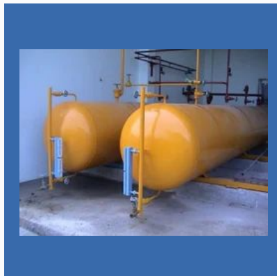
Ammonia High Pressure Receiver
