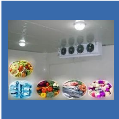
pharma cold room
