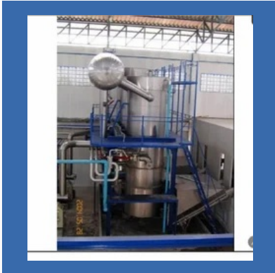
Ammonia Tube Ice Plant
