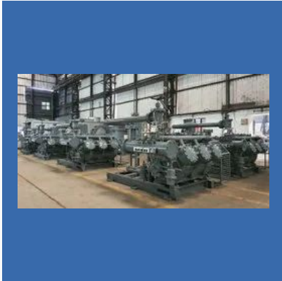
Ammonia compressor packages.
